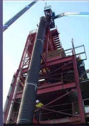
Continuous Leach Vessel
