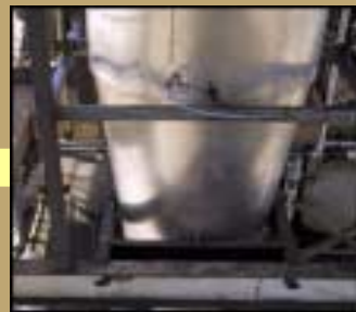
EARS acid regeneration plant
