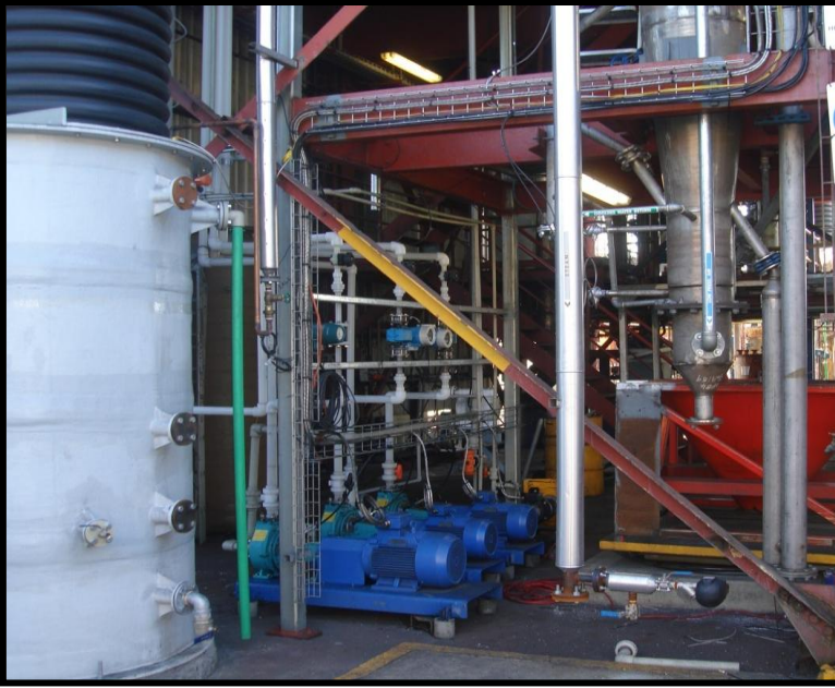
Base of Continuous Leach Reactor and associated piping and pumps.
