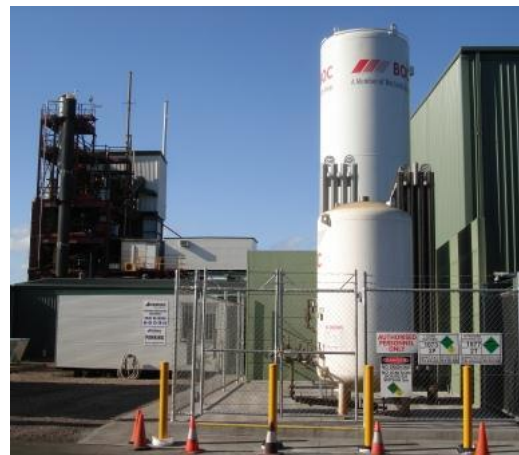
New nitrogen and oxygen gas storage area
