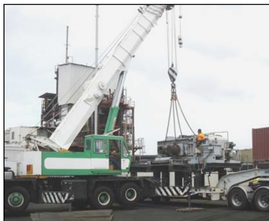
Delivery of the Koeppern briquetting press to the Newcastle Iron Recovery Plant.
