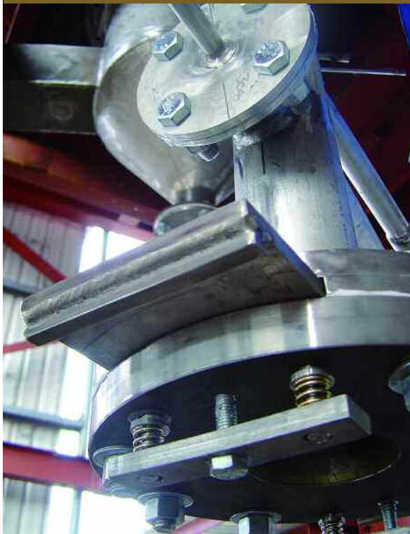
High temperature solids isolation valve
