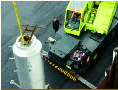
Installation of ERMS afterburner
