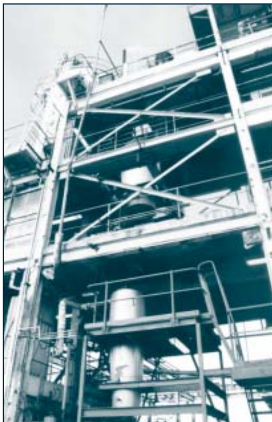
The ERMS SR oxidation and reduction roasting train occupies five floors of the pilot plant
