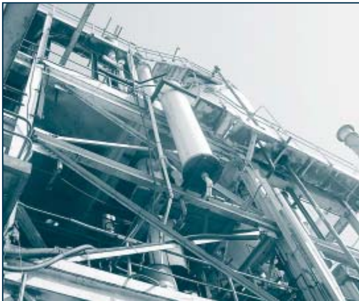
EARS acid regeneration absorption columns at Kooragang Island pilot plant
