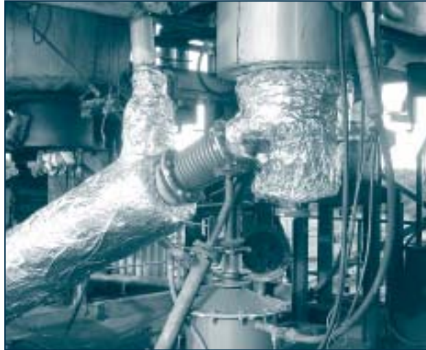
LTR gas feed system and anaerobic solids cooler
