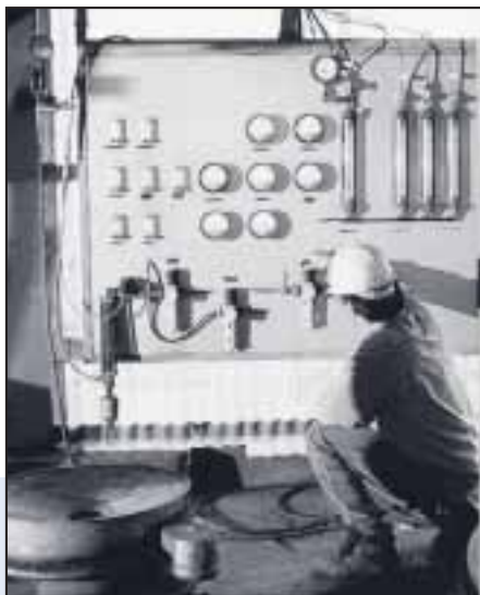
Centralised pneumatic control centre at the pilot plant
