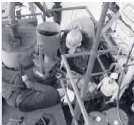
Calibration of ilmenite feed to pre-heat reactor
