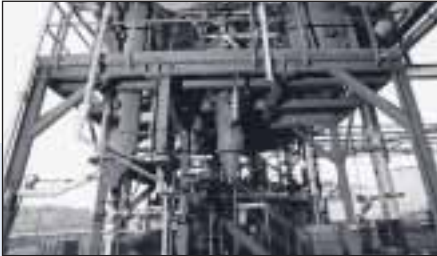
Leaching section of the pilot plant
